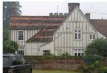
The likely positions of the timber frame elements, based on the thermographic survey are shown overlaid on the photograph.
