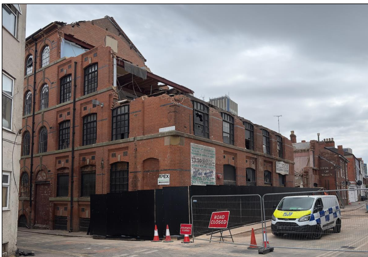
Figure 1: The damaged building on the corner of Wharf Street South and Wheat Street (photo: Colin Hyde)
