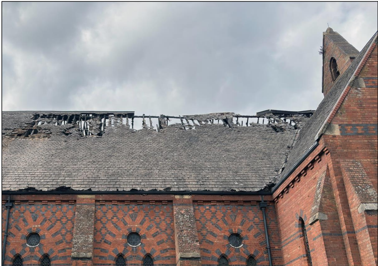
Figure 5: Damage to the roof of St Andrew's Church as seen from Jarrom Street (photo: Colin Hyde)
