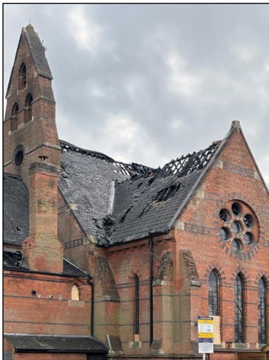
Figure 3: Damage to the exterior (photo: Colin Hyde)
